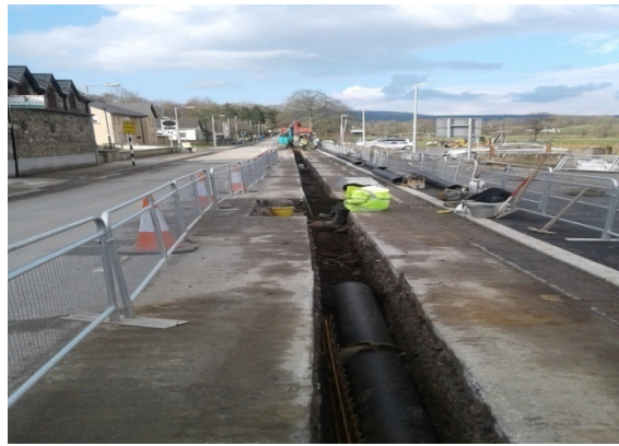
Trench works in the village of Inistioge, Archaeologist mapping portion of town wall/ gate.
