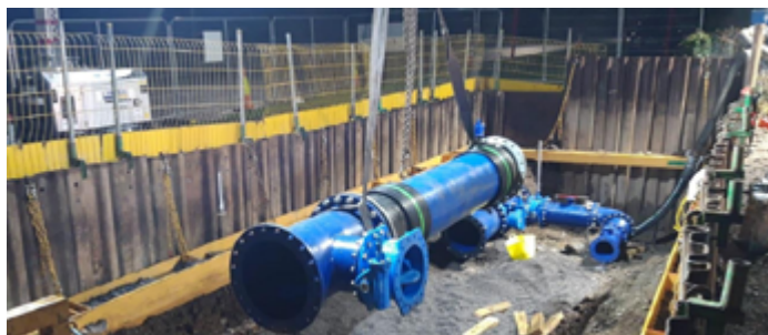
PRV installation at Radestown WTP
