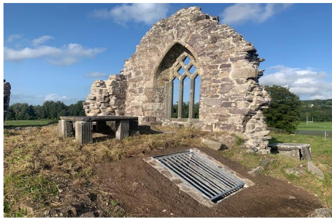
New gate installed at the entrance to the underground vault at The Thomple Historic Church & Graveyard
